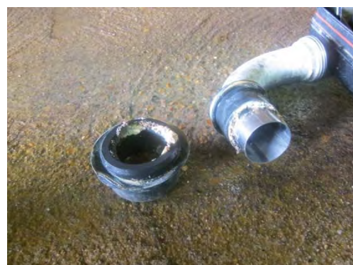
Figure 3 : Raccord encrassé (source personnelle)
